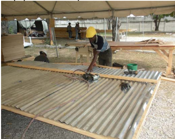
3. Pneumatic tools are being used in the shop to apply the corrugated galvanized iron for the walls.
