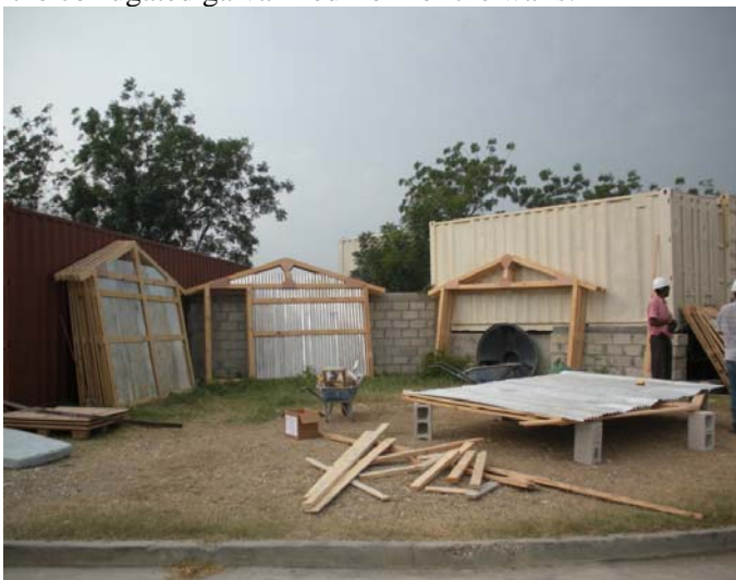
5. View of the three different prefabricated panels. All three sections are ready to be transported.
