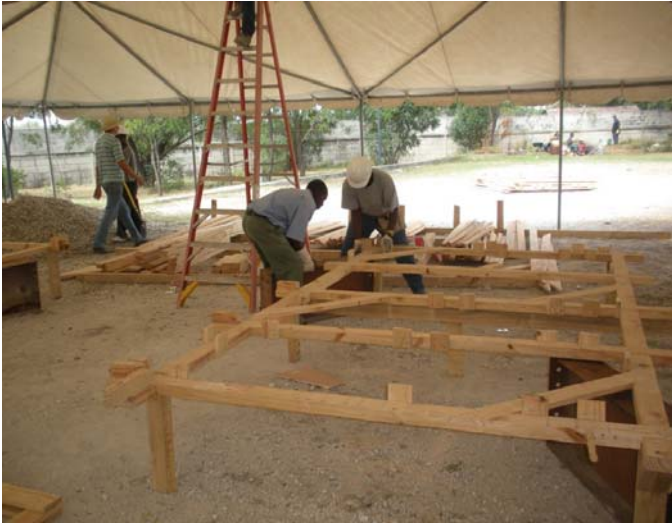
1. Fabrication shop for transitional shelters. Jigs were prepared for the end panels.
