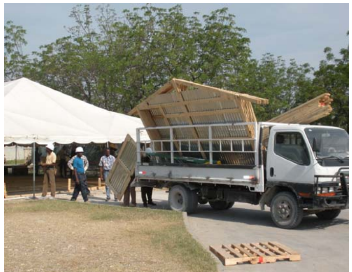
6. First truckload of prefabricated panels and materials being loaded for delivery to their destination.
